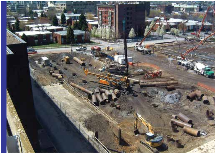
The mines below the building didn't allow the complete structure to be four stories tall. Here the east side is built on a mat slab, which required a 22-hour continuous pour of cement.
